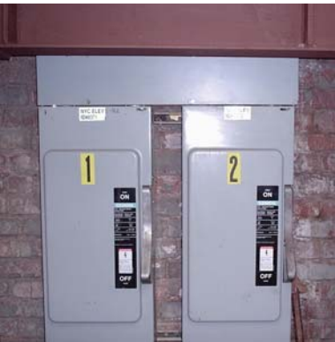
Two Elevator Fused Disconnects
