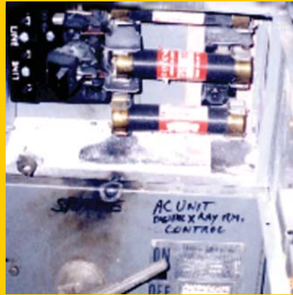
Opening of a Defective Disconnect With Screwdriver
