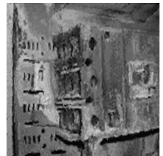
Remains of Breaker After Catastrophic Failure
